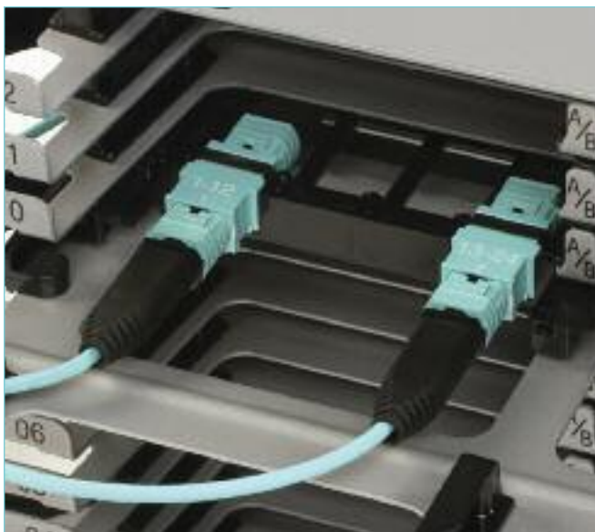
Pretium EDGE Solutions MTP Connector Panel Installed in Housing | Photo LAN1694
