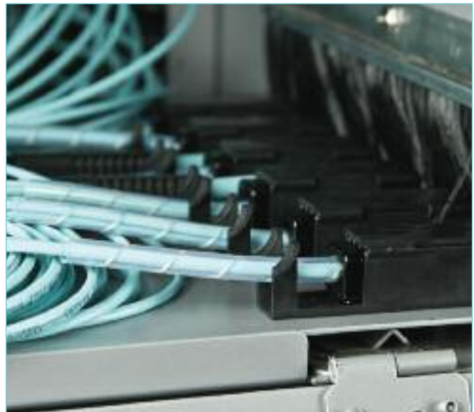
Pretium EDGE Solutions Trunk Integration | Photo LAN1748
